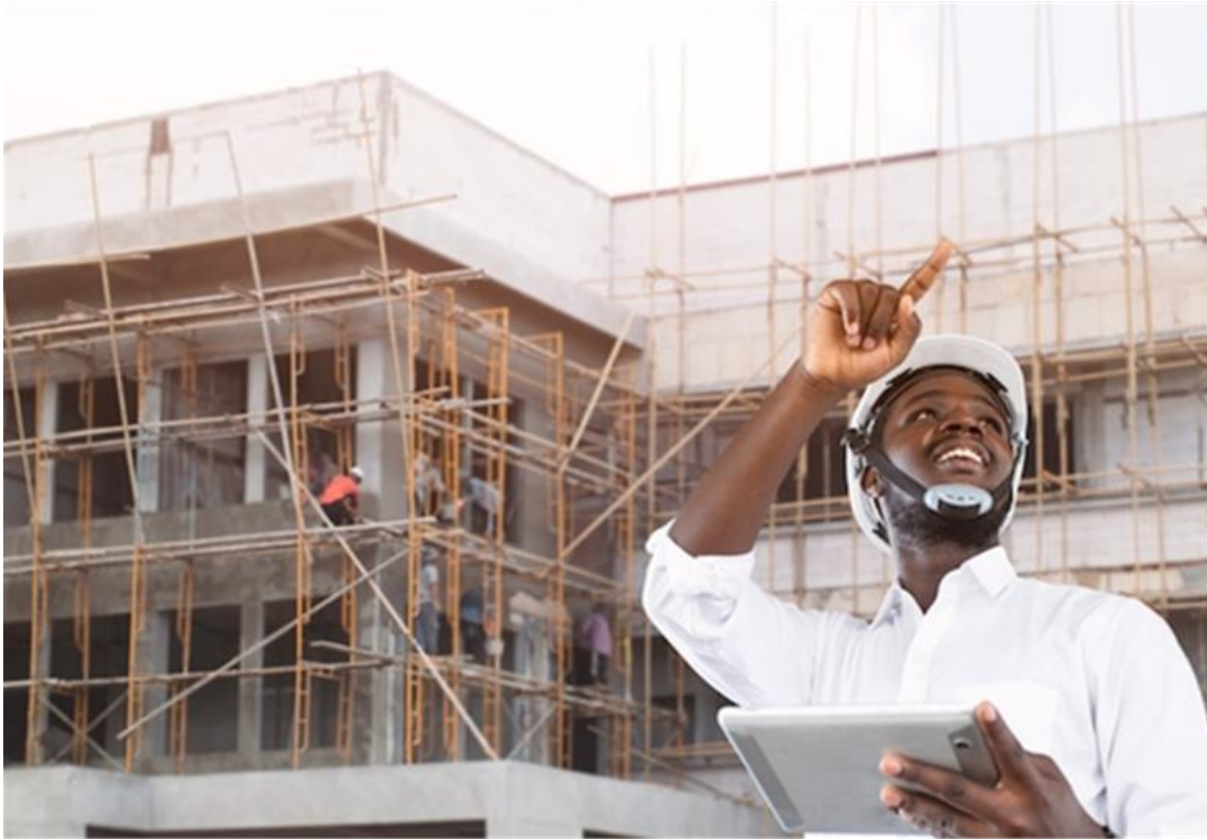
Figure 4. 3 : Site contractor engineer with hard hat holding tablet with the building in background.
