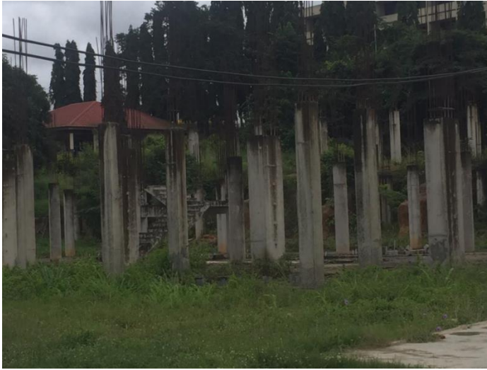
Figure 4. 7 : Results and discussion of observation at cape coast Technical University the researcher observed the following from the university are the Abundant School Building auditorium on construction site due to poor communication and planning
